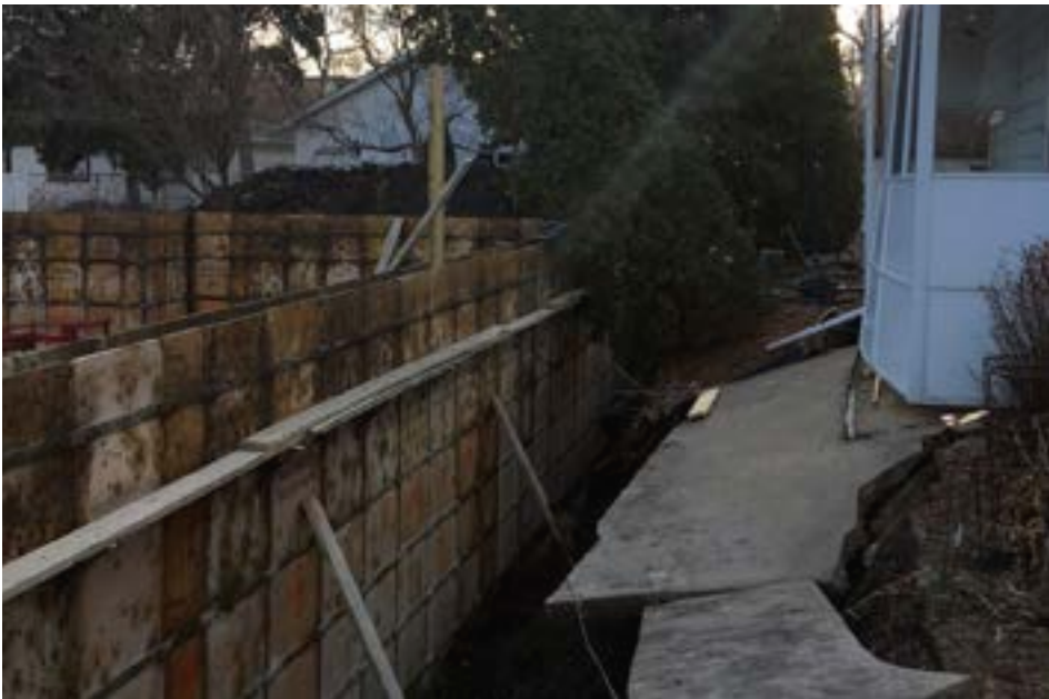
Collapsing excavation on 110 St.
